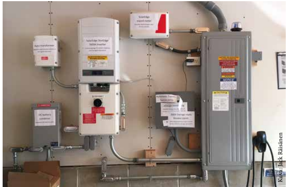
Kukkonen's garage wall has a variety of electrical equipment to manage the energy flow of solar panels, storage batteries, and chargers. Everything was well-marked to show visitors.
