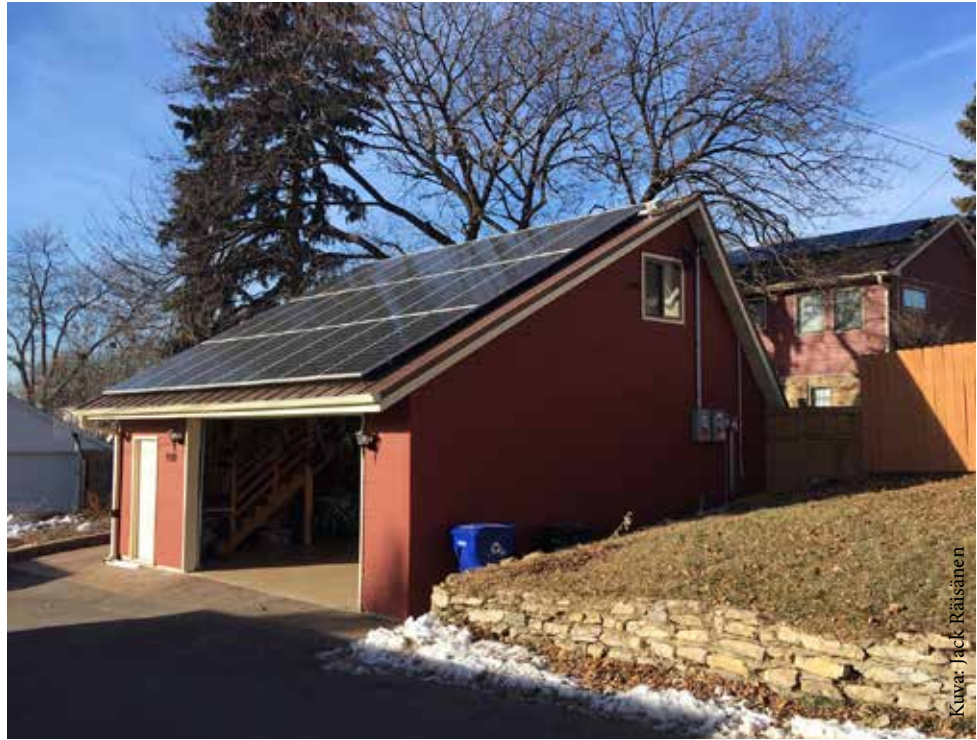
Solar panels on Kukkonen's home and garage produce electricity for household needs, car charging, and sometimes even selling back to the grid.
